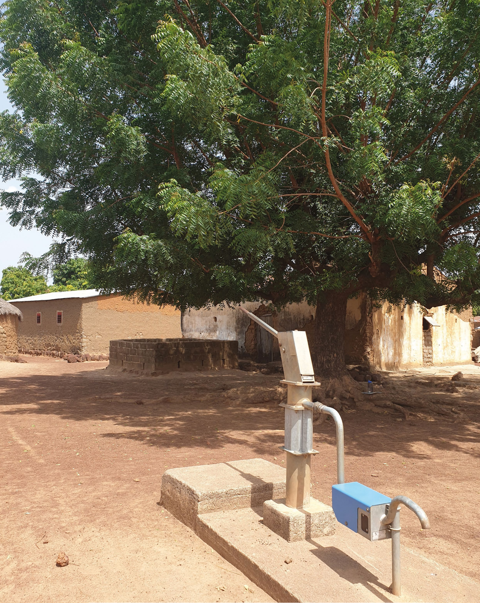
India Mark 2 handpump in Tiefala, Mali. Photo by Johannes Wagner.
